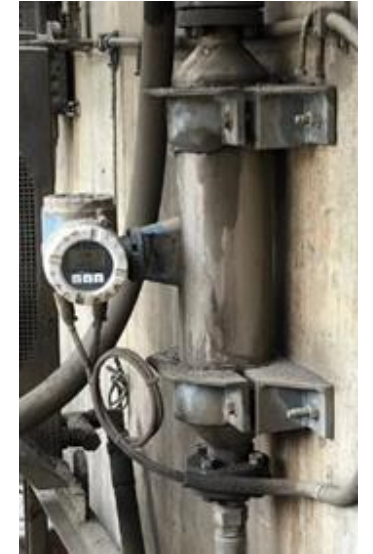
Promass I 300 installed in the field
